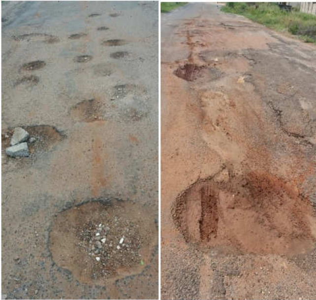
Figure 1: Potholes and Road Obstacles
